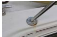
Rust at or on fittings
