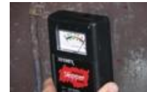
High moisture content
