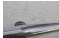
Cracks in gel coat at stanchion
