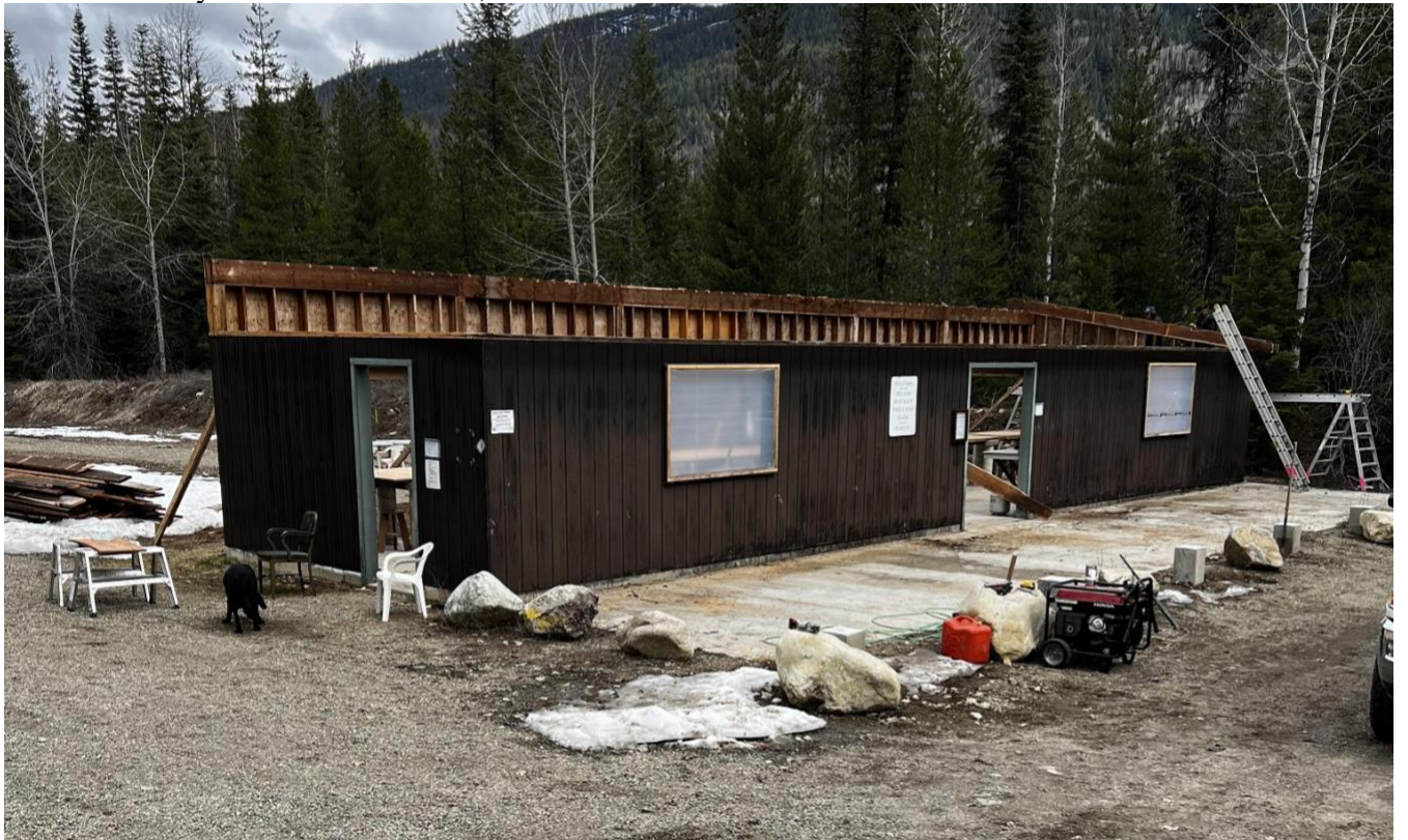
Then Ryan Coates and Crew, with NDRGC Volunteers Demolished the old structure:
